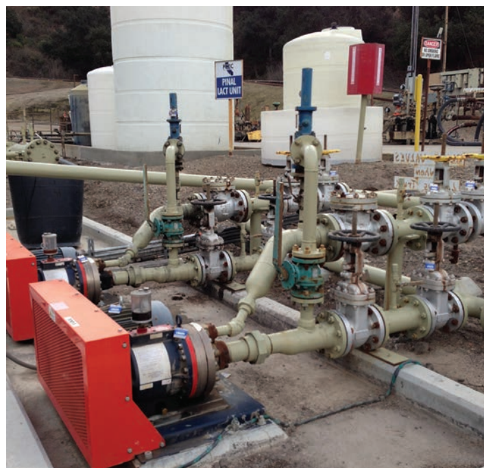
Hydra-Cell pumps shown processing volatile crude oil.
