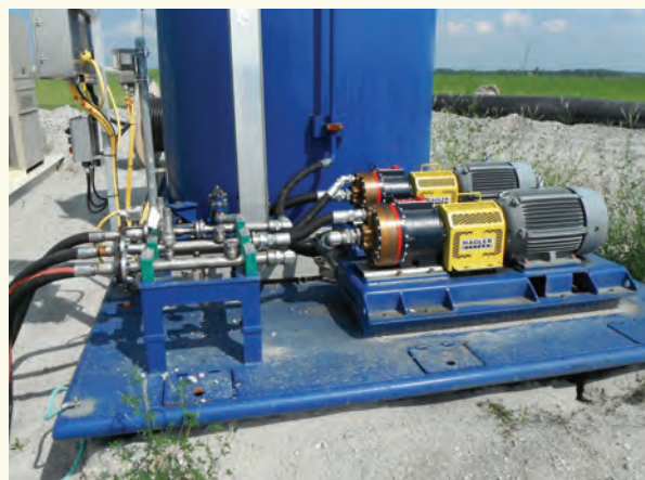
Gland seal flushing for a Haglar Systems customer.
