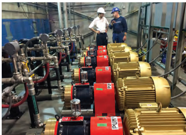
Hydra-Cell D35 model pumps used at a manufacturing facility for the removal of welding slag and cleaning of a conduit pipe.
