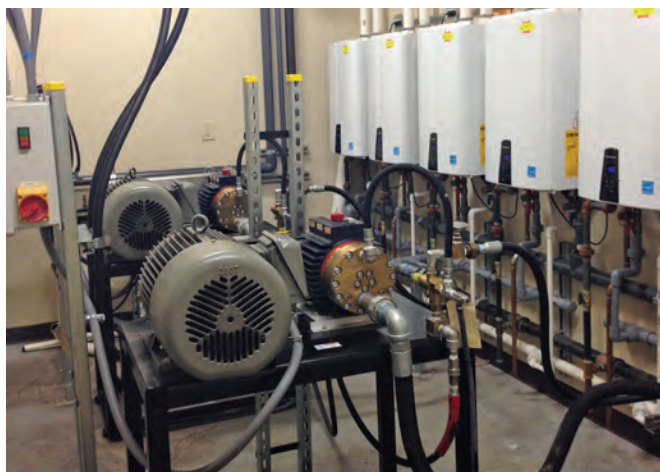
Hydra-Cell D15 model pumps used for high-pressure wash down at a meat processing plant.
