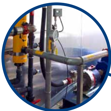
Sea and high brackish water desalination
