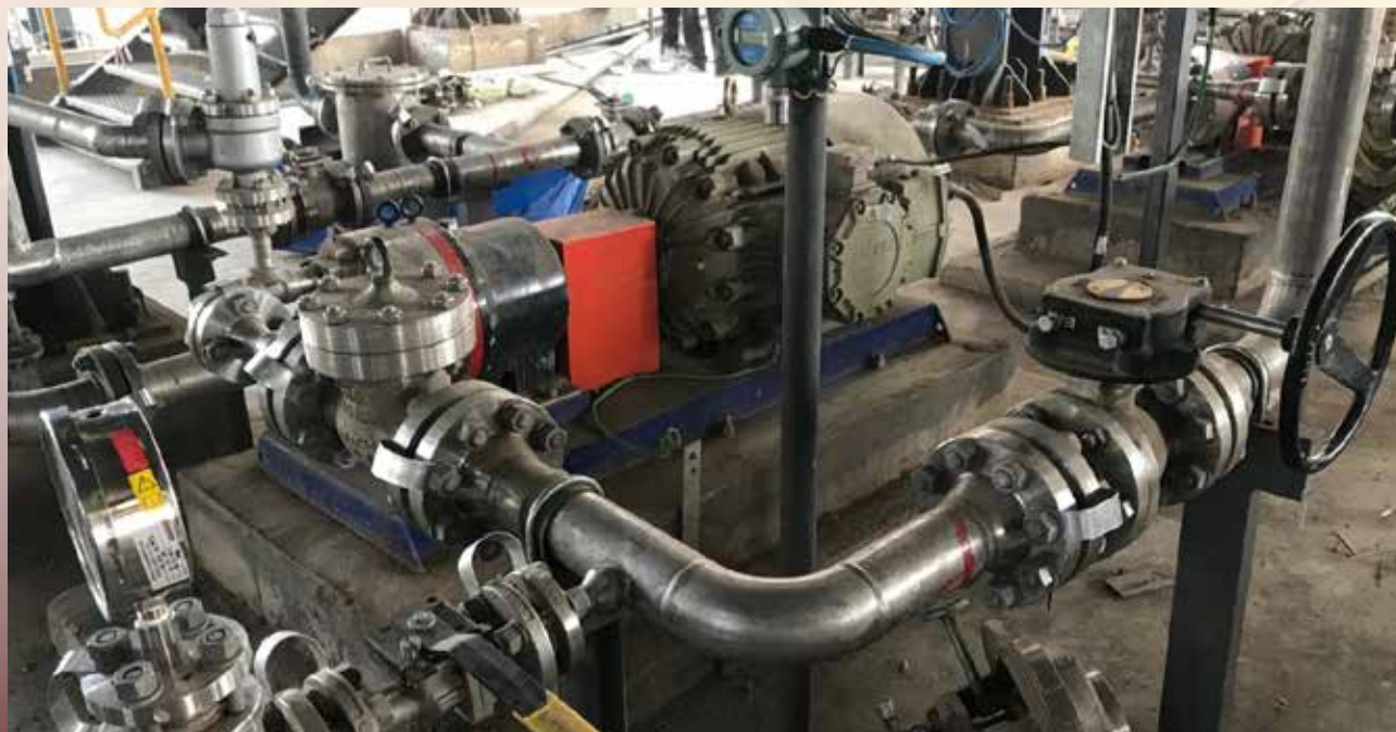
Methanol injection pump
