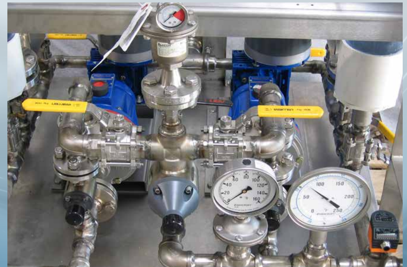
Polymer dosing for water treatment
