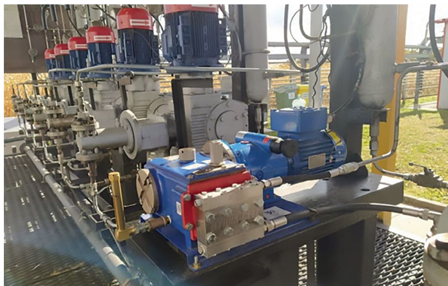
A metering pump in-situ
