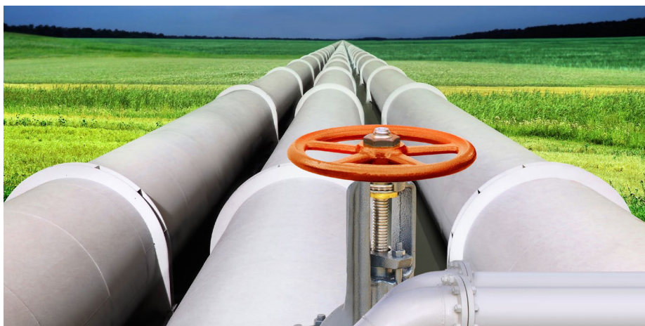
A gas transmission pipeline
