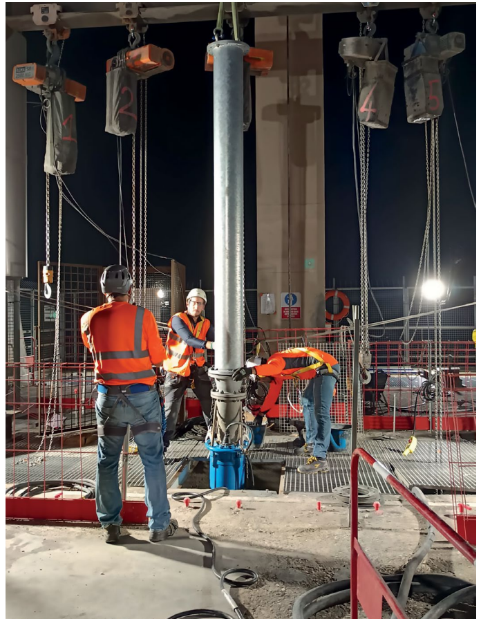
Installation of a pipe extension for a height difference of 21 metres. Picture from Tsurumi
