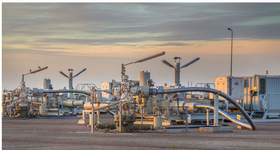
A natural gas production plant with pipeline valves
